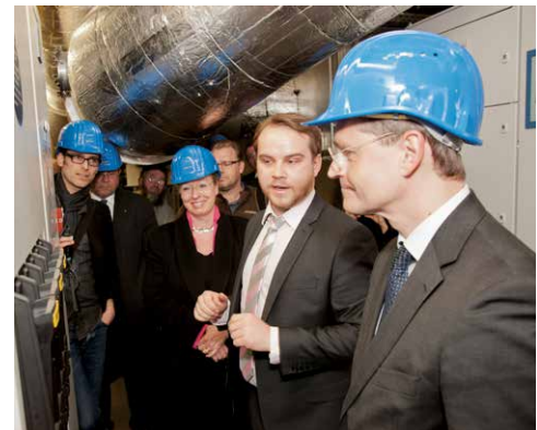
White City, a UNESCO World Heritage Site, has been supplied with heat and power by its own CHP unit since April 2012. © Fotoarchiv der Deutsche Wohnen AG
